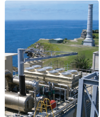
Remote Community Power Stations
