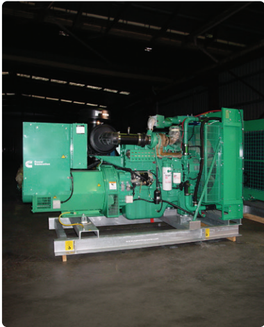
Skid Mounted Pump & Gensets
