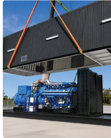
Data Centre Standby Gensets
