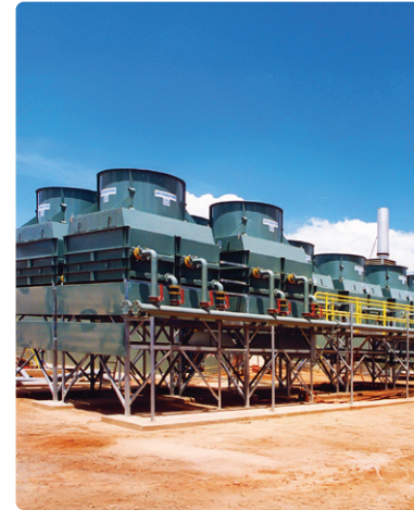
Mine Site Power Stations
